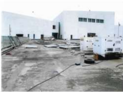
Plate 1: Vandalized Calabar International Conference Centre
