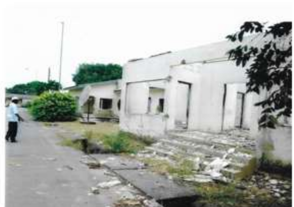
Plate 4: Vandalized Vehicle Inspection Office (VIO) at Ekorinim
