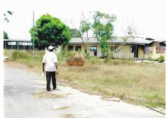
Plate 6: Vandalized Training School Ministry of Work at Ekorinim
