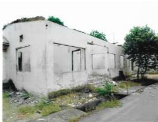
Plate 9: Vandalized State Electrification Agency, Ministry of Works, Ekorinim
